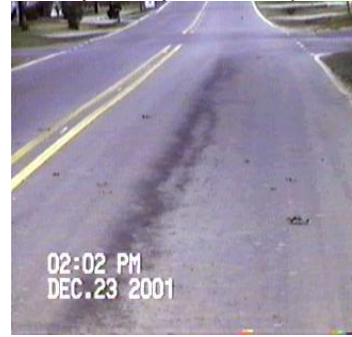
Leachate on roads
